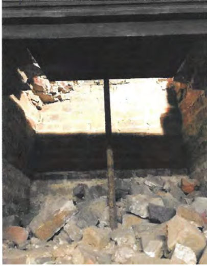
Underside of the paneled room fireplace, showing the steel sheet and its support. Photo by Virginia Masonry.
