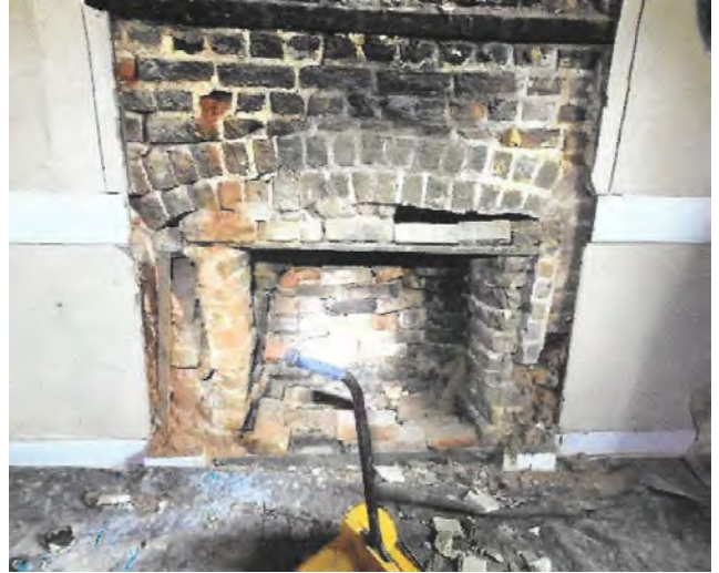
North ell fireplace, minus the mantle and surround. Photo by Virginia Masonry.
