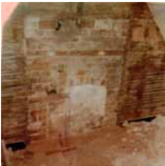
▲ Figure 3. Bricked in fireplace. Note stripped lathing and shadow of the original mantel.
